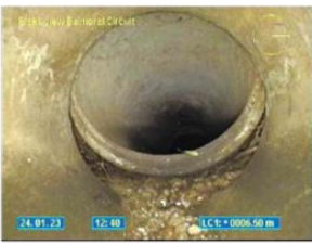
Pipe requiring renewal works
