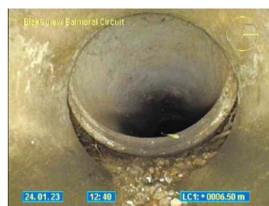
Pipe requiring renewal works
